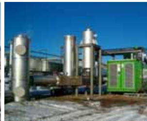
Exhaust Heat Recovery System
